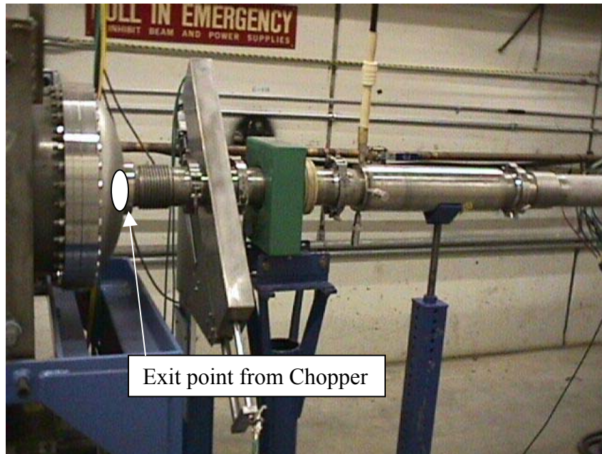
Figure 3. Area downstream of the Chopper. The Wire Scanner and the Transformer can be moved downstream. The downstream cover on the Chopper will have to be modified to allow the insertion of the downstream pulsed magnet with the two beam pipes as indicated in figure 1
